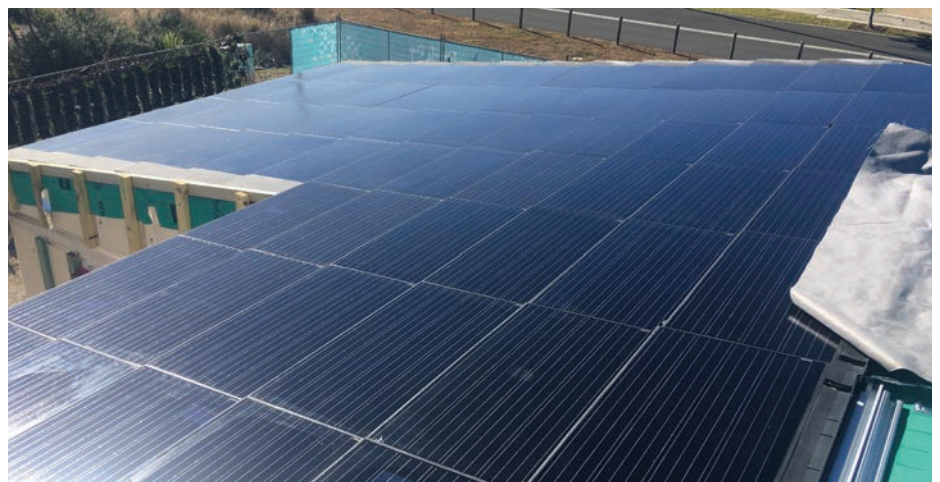
Figure 2.40 - BIPV-T Installed on Desert Rose Roof
