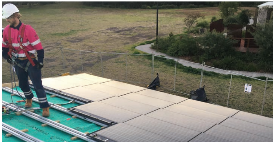
Figure 2.32 - Team UOW Assembling the BIPV-T on the Roof of the Desert Rose
