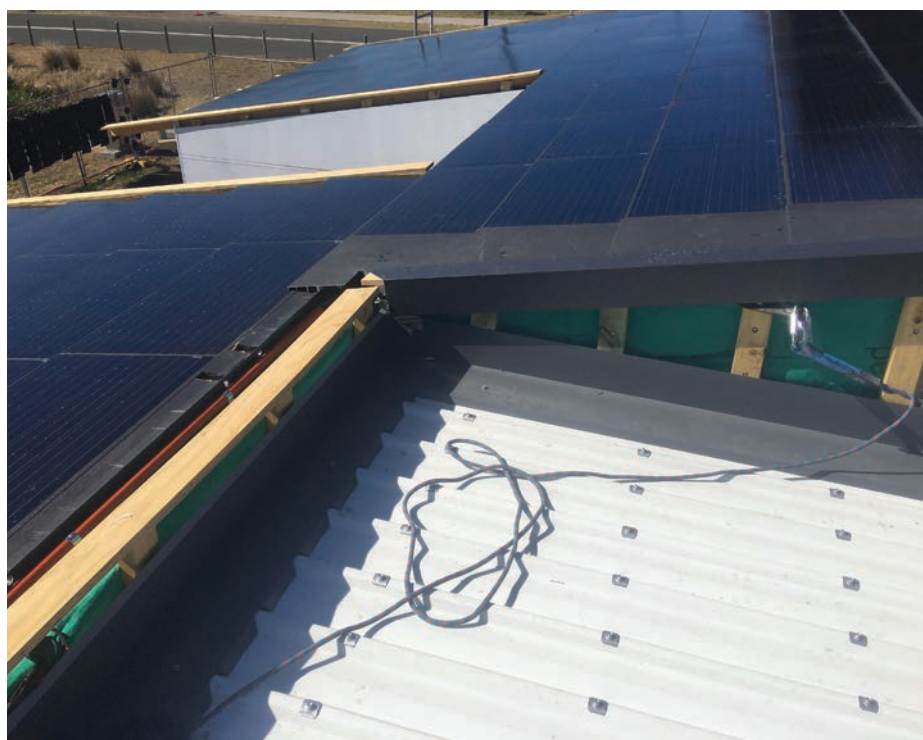
Left: Figure 2.4 - Clerestory Windows Above Kitchen and Dining Area Above: Figure 2.5 - BIPV-T and Coolmax Sheeting on the Roof of the Desert Rose
